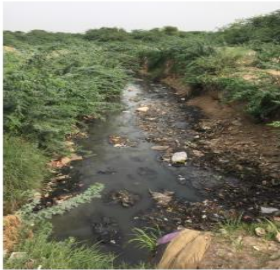
Natural drain carrying domestic sewage (RUIDP)
